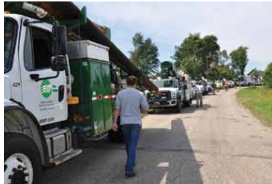
Far left: Approximately 50 poles needed to be replaced due to storm damage.
